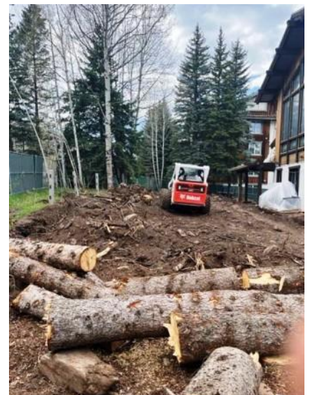
Unauthorized Tree Removal
