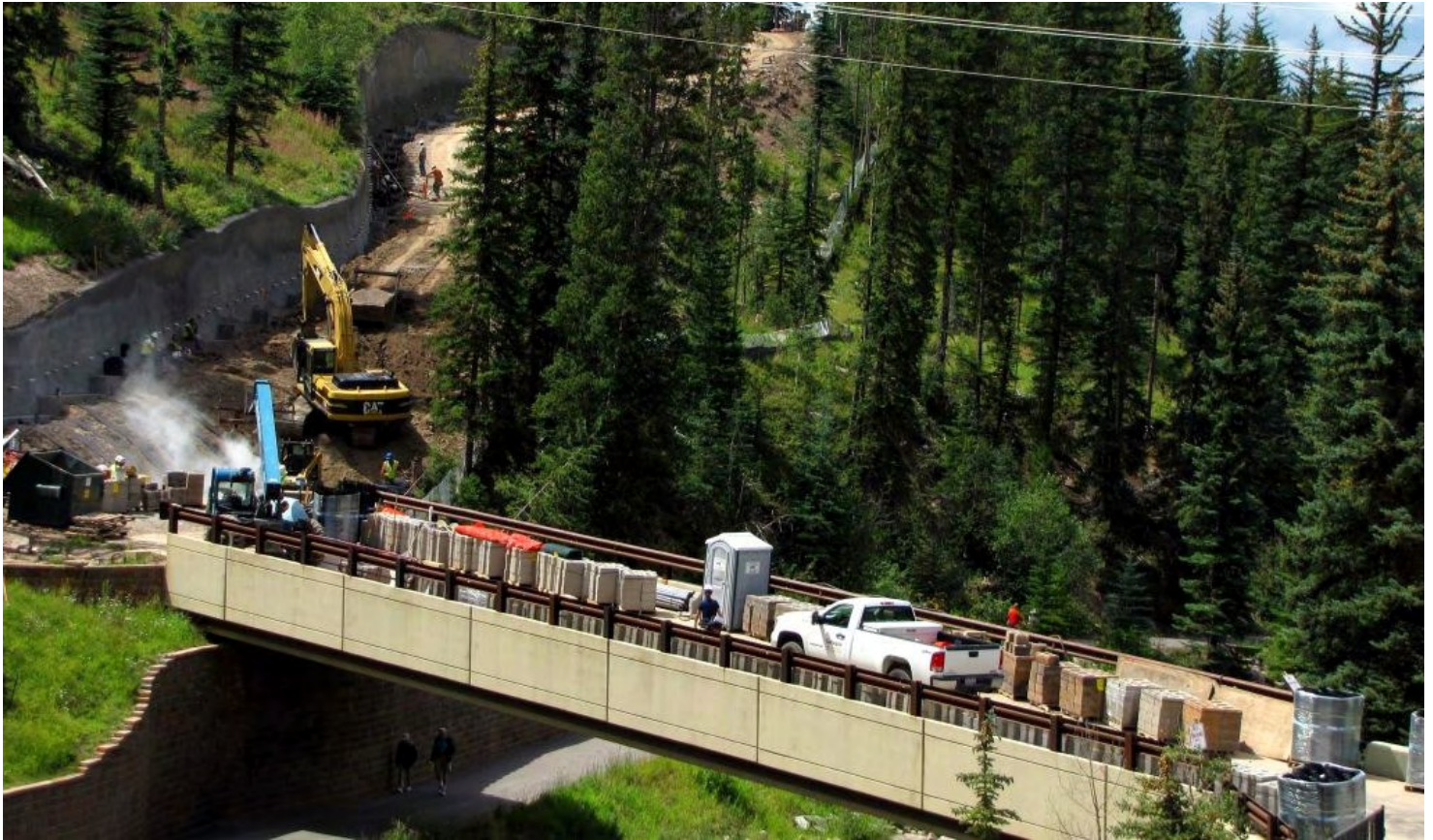
New Vail Mountain snow cat access route under construction in West Lionshead.
