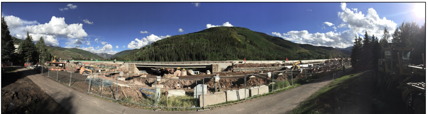
Simba Run Underpass is taking shape. The carrying capacity of Vail’s central boulevard is being extended by 20 years.
