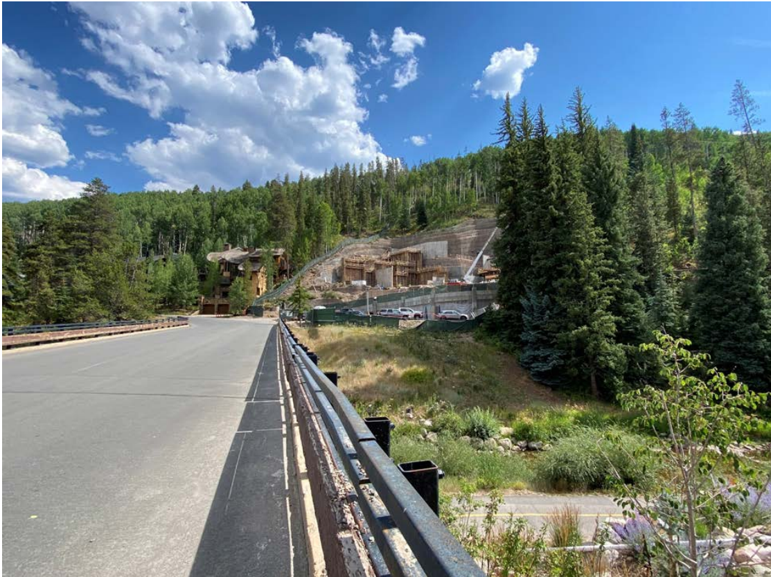
Project under construction on West Forest Road near Gore Creek located upstream of the community's nearby waste water treatment plant.
