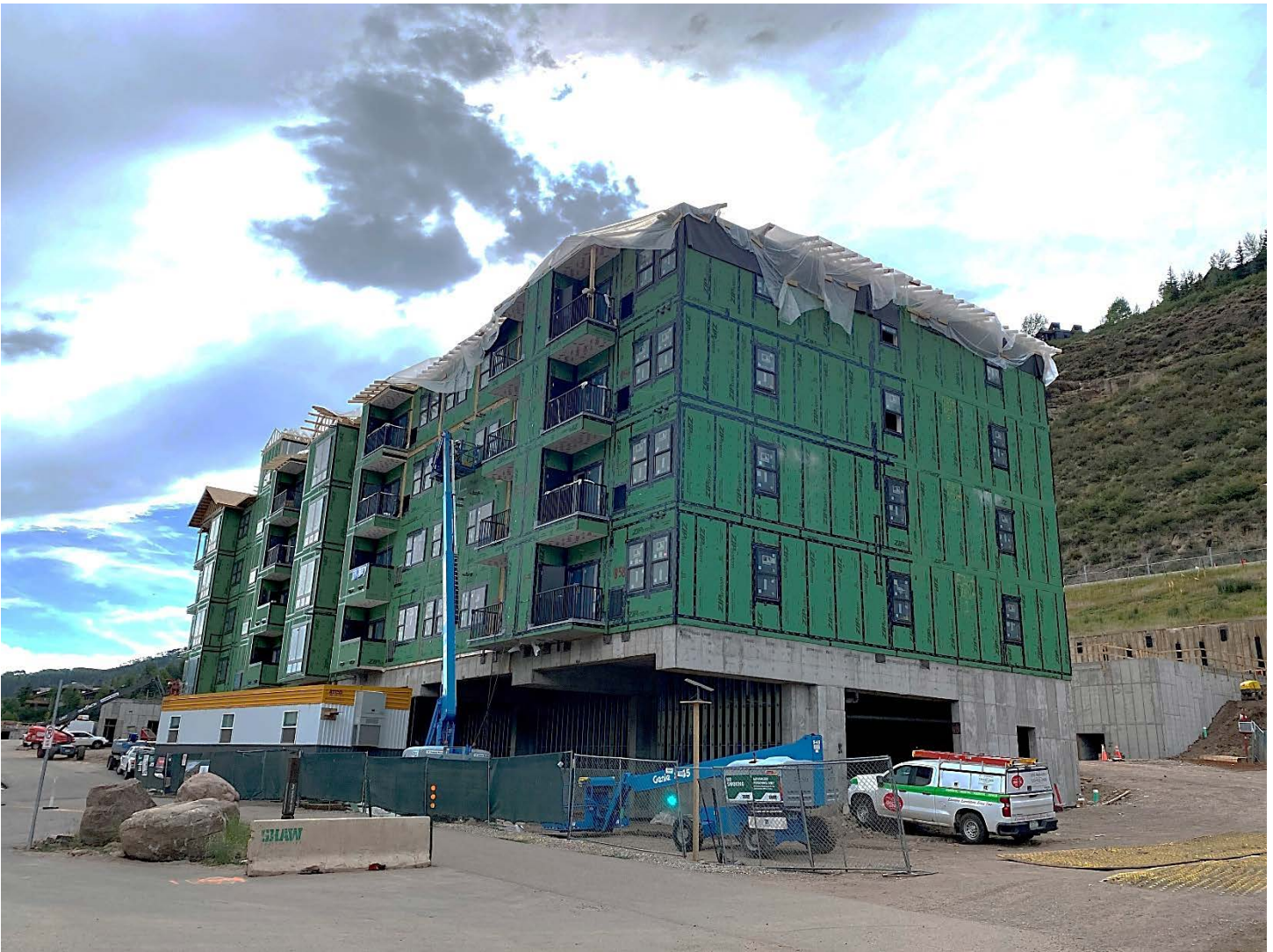
West Timber Ridge - The first of seven residential apartment buildings under construction in West Vail.
